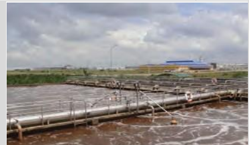
Wastewater Treatment System in Industrial Zone
