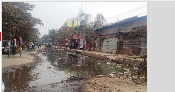
Deteriorating roads and lack of storm water drains
